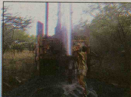
This is what 144,000 liters per hour looks like while drilling for water
